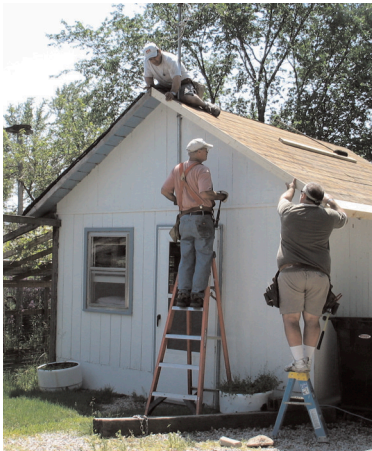
Bob Rose (lt) & Dale putting a new roof on the kitty cottage.
